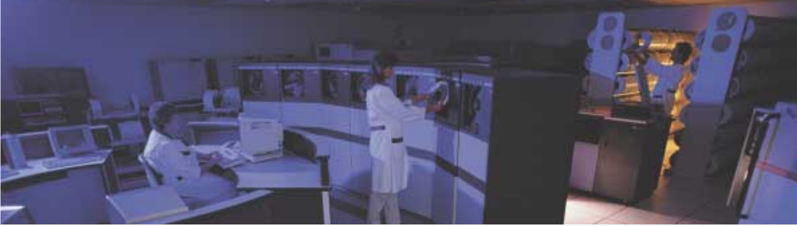
Data centre: Security application
